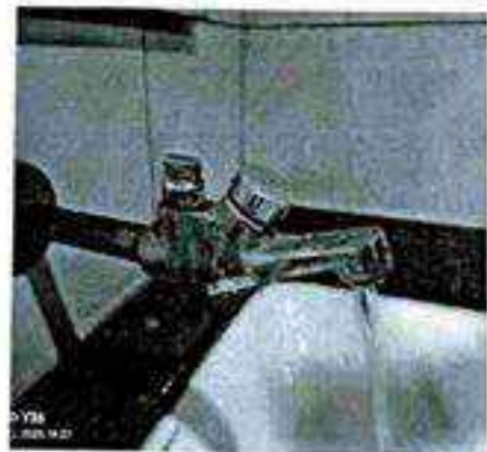
Tap water flow rate monitoring
