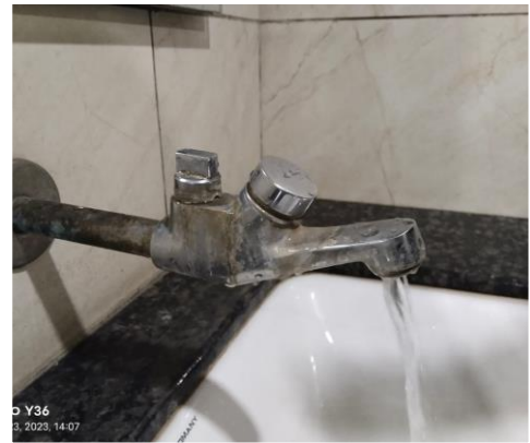
Tap water flow rate monitoring
