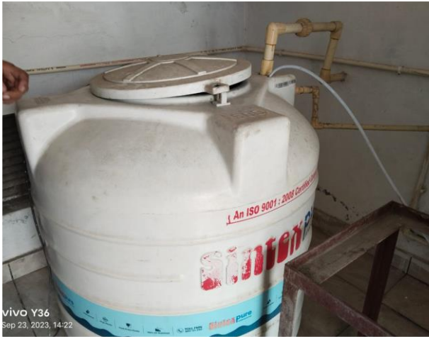
RO Wastewater collection tank
